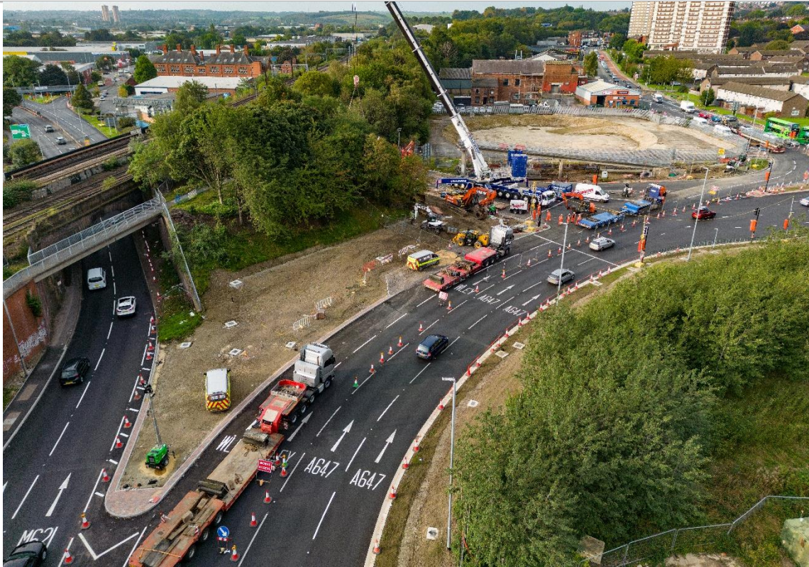
Specialised removal vehicles wait to remove the old bridge beams from site.
