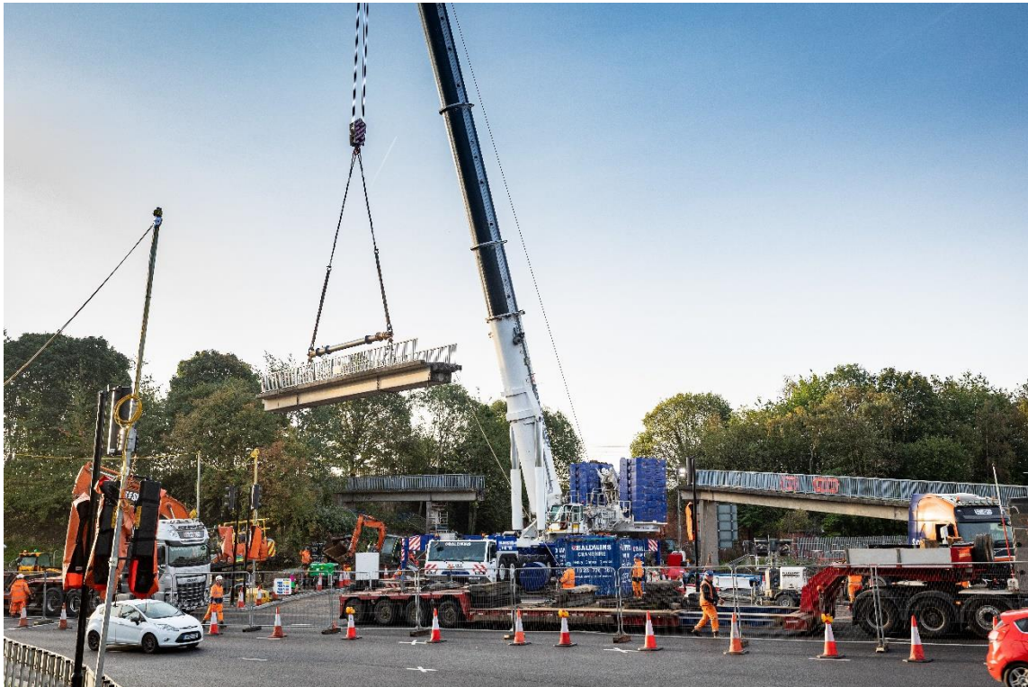
One of the post tensioned concrete beams that formed part of the Spence Lane Footbridge being removed.
