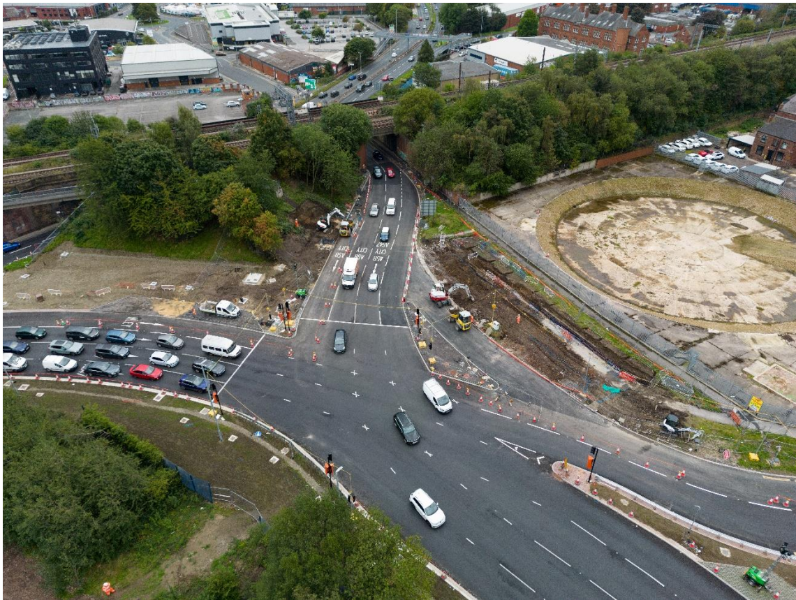
Ingram Distributor (north bound) without a footbridge, ready for construction to begin on the new one.
